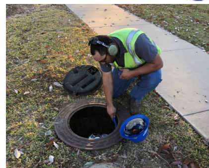
Another utility employee uses acoustical leak detection equipment on a water valve.
